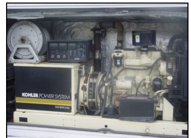
30KW Generator and powered cord reel offers service with or without benefit of shorepower
